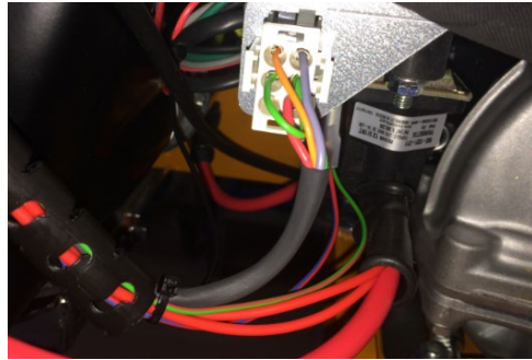
Orange shut-off valve carburettor Green oil pressure switch
