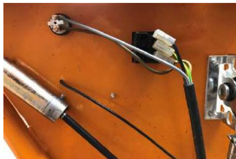
AS 701 cabling – handlebar with old start switch.
