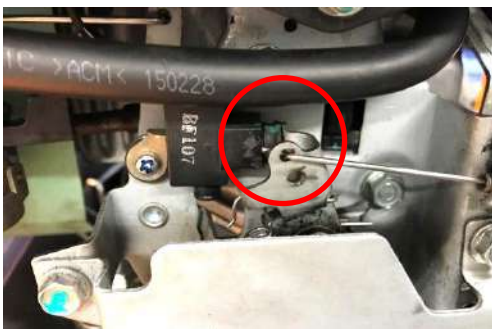
Position of the accelerator cable at "off". Throttle lever touches and switches the short-circuit contact.
