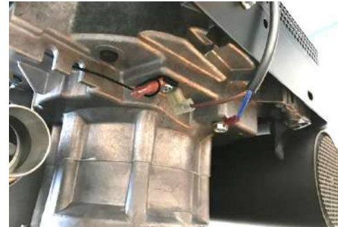
Cabling on the engine.
