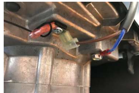
Cabling on the engine. The black cable with the red plug is the short-circuit cable of the electronic ignition.
